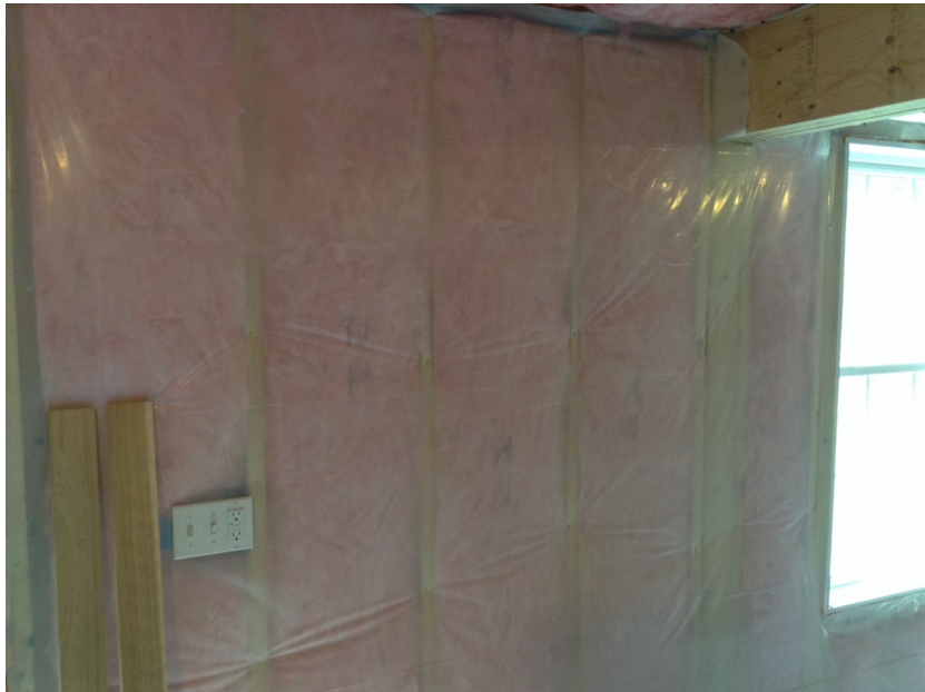
Figure 35: Grade II Fiberglass Batts – Basement Walls
