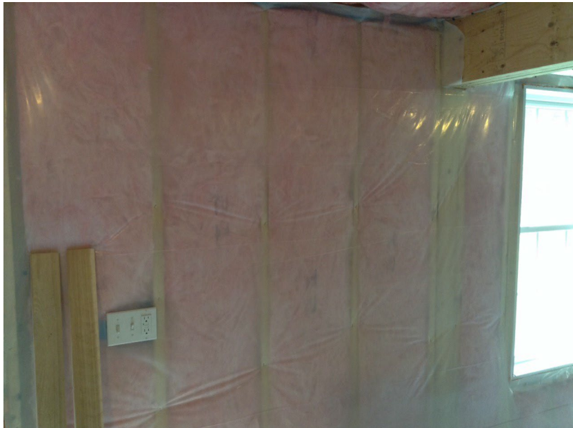
Figure 36: Grade II Fiberglass Batts – Basement Walls
