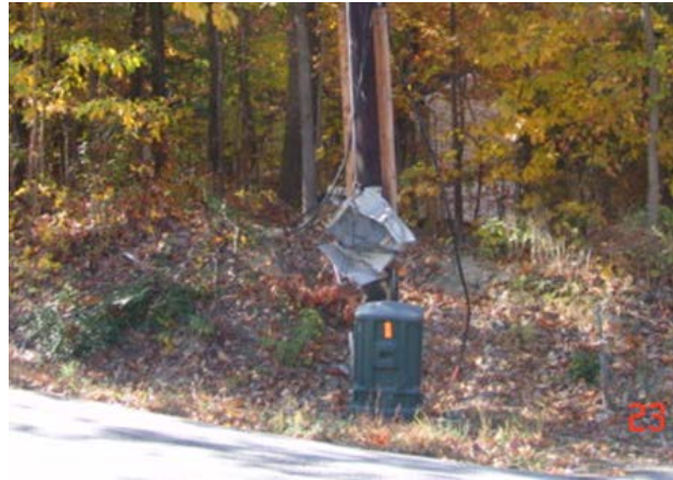
Verizon's picture showing box and pedestal
