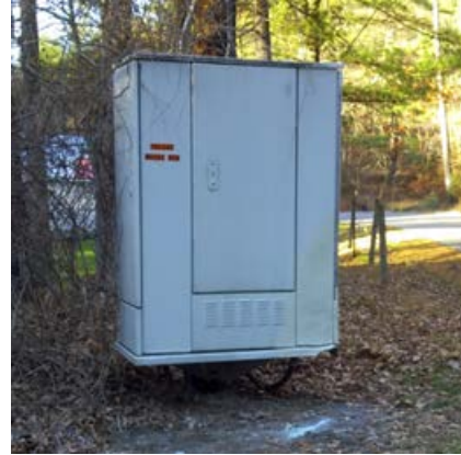
Verizon picture 11/3/15 Shows cabinet repaired
