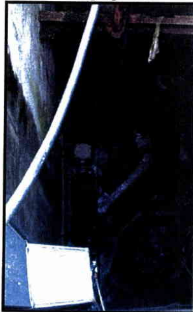
Comminutor/Bypass Channel Photograph 6.1
