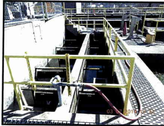
Chlorine Contact Tank Photograph 6.4
