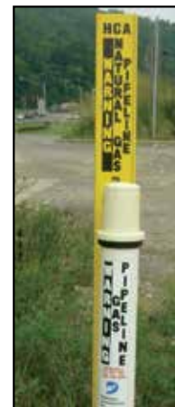
5. HCA marker and cathodic protection test station
