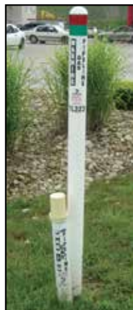
2. linemarker and cathodic protection test station
