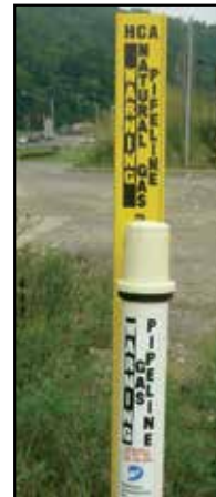
5. HCA marker and cathodic protection test station
