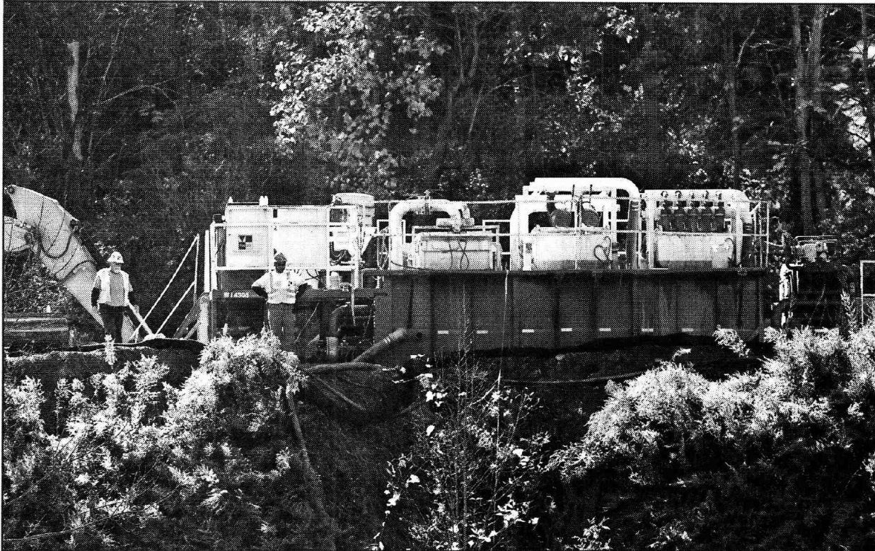
Columbia Gas workers installed a new pipeline last year in Emlenton Borough. Crews worked on the south bank of the Allegheny River under the Interstate 80 bridge in October. The new line replaced about 1,500 feet of old gas line under the Allegheny River.
