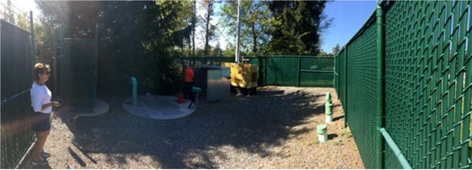
Pump Station #4 – Fernridge
