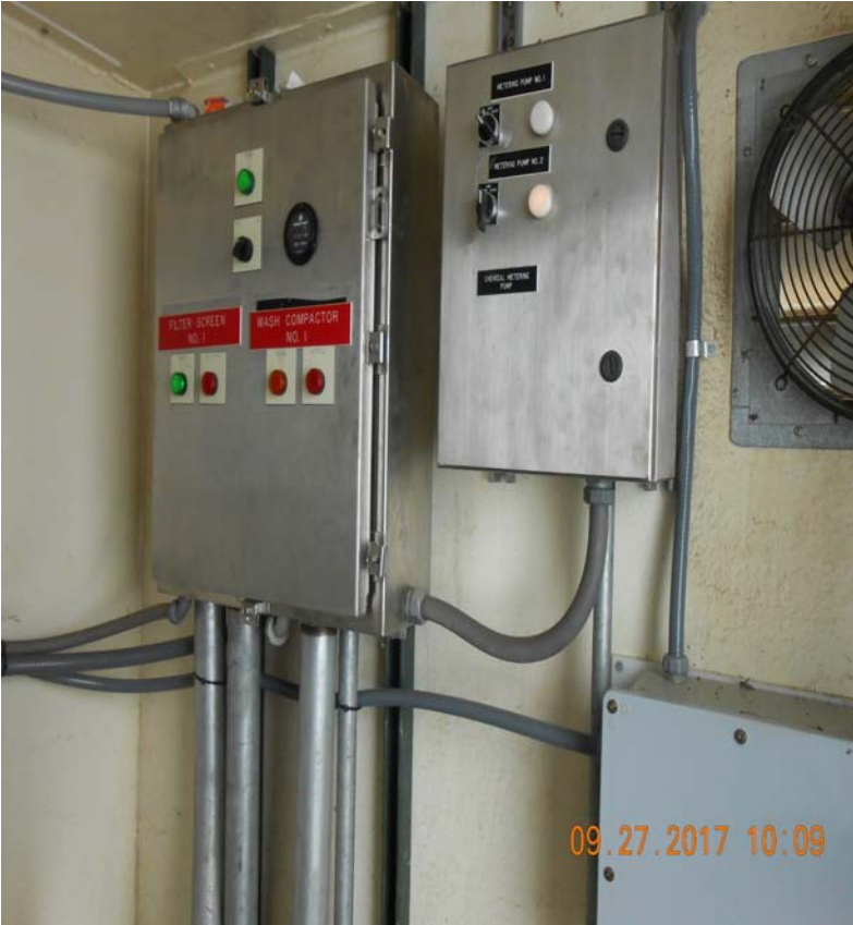
Control Panel for Submersible Pumps
