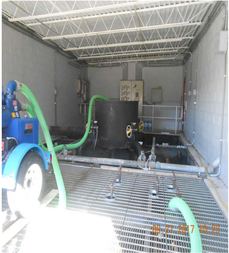
Back Wash Pumps
