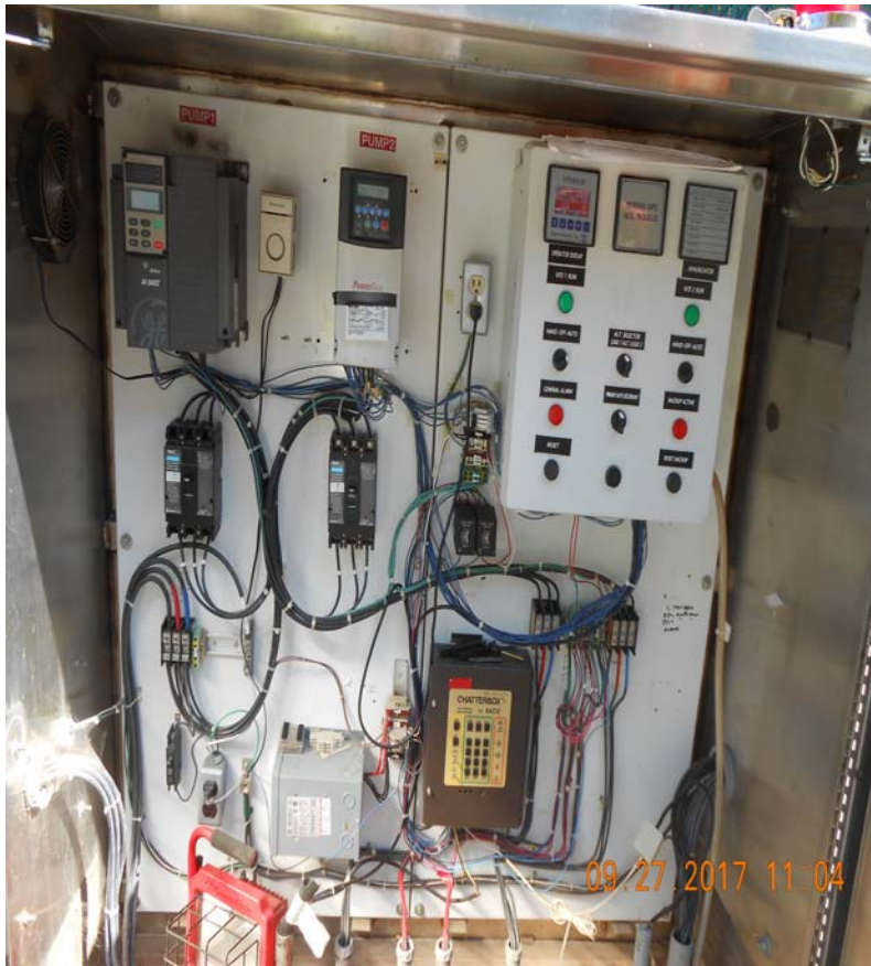
Control Panel for Greenwood Pump Station
