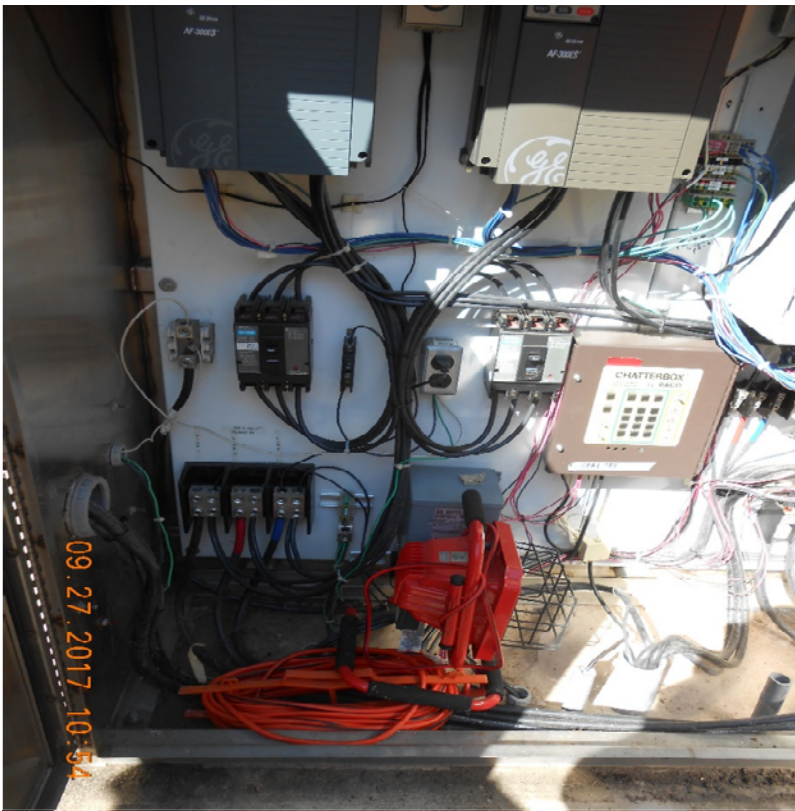
Control Panel for Pump Station #1
