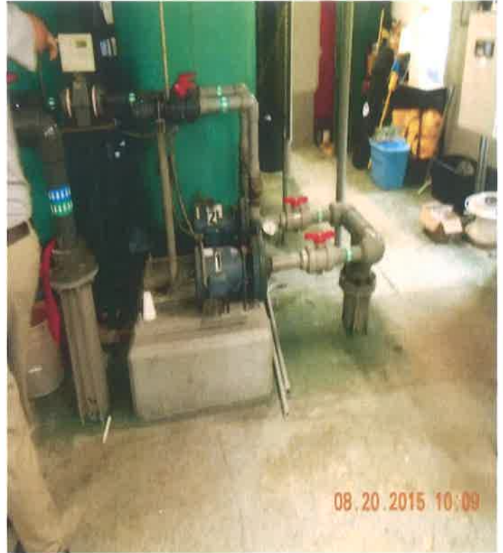
Membrane Filter and Pumps
