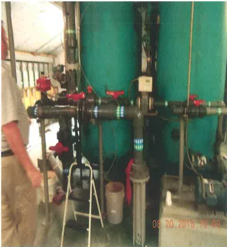
Membrane Filter and Pumps
