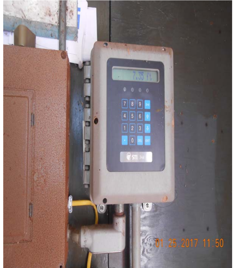
Interior Well House # 1
