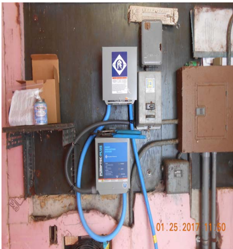
Interior Well House # 1
