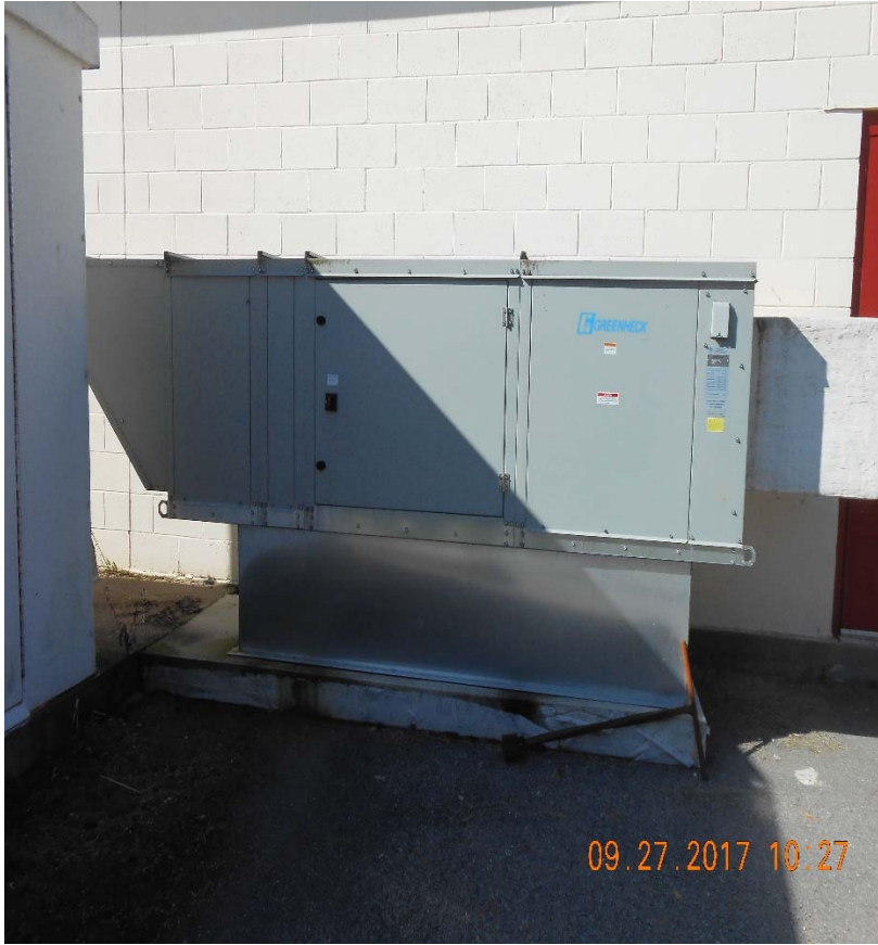
Heaters for Blowers
