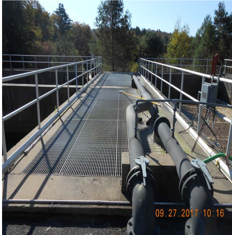
SBR Screened Tanks
