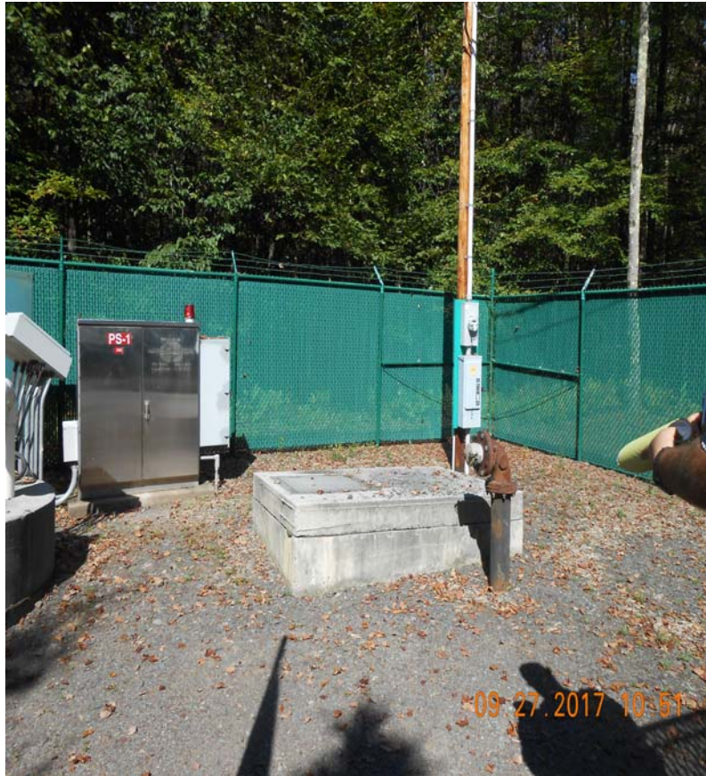
Pump Station #1 – Lady Jennifer
