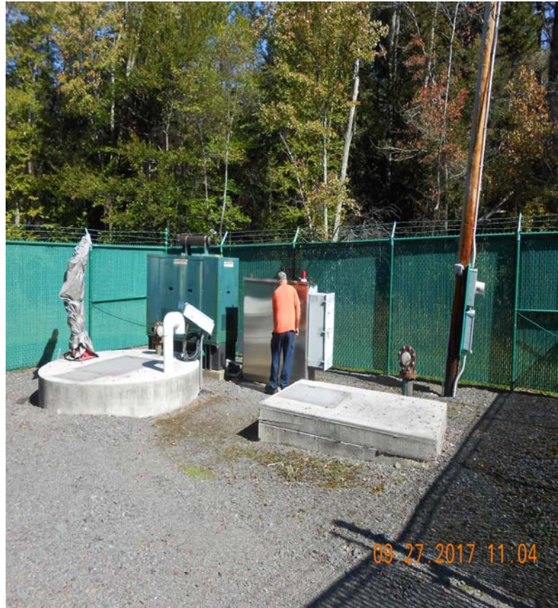
Greenwood Pump Station
