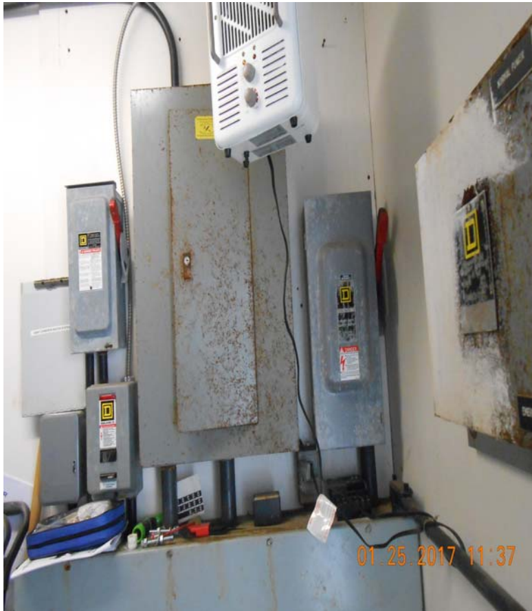
Well # 2 Control Panel
