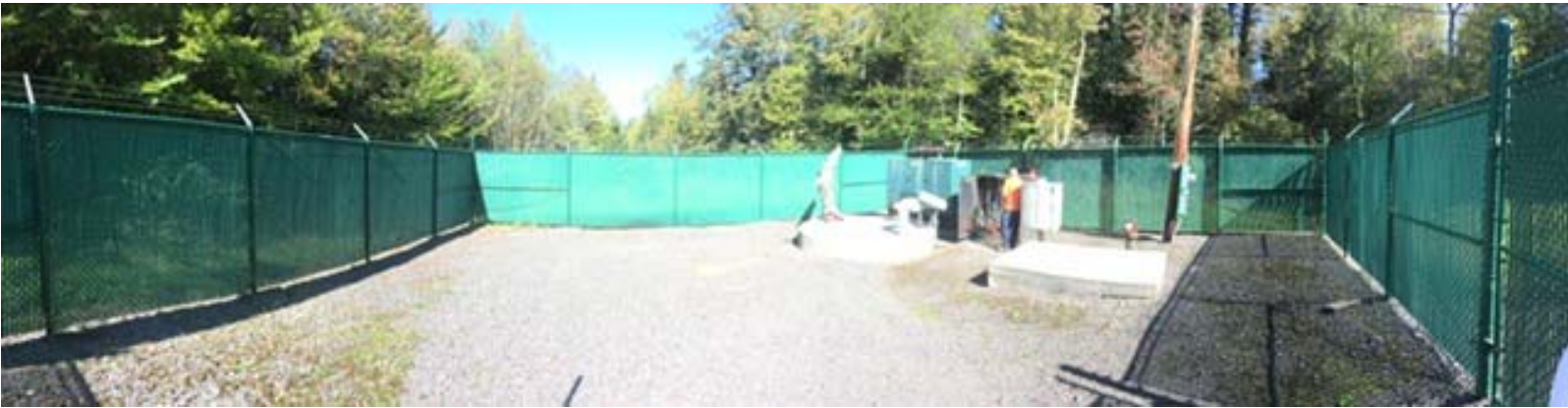
Pump Station #2 = Greenwood
