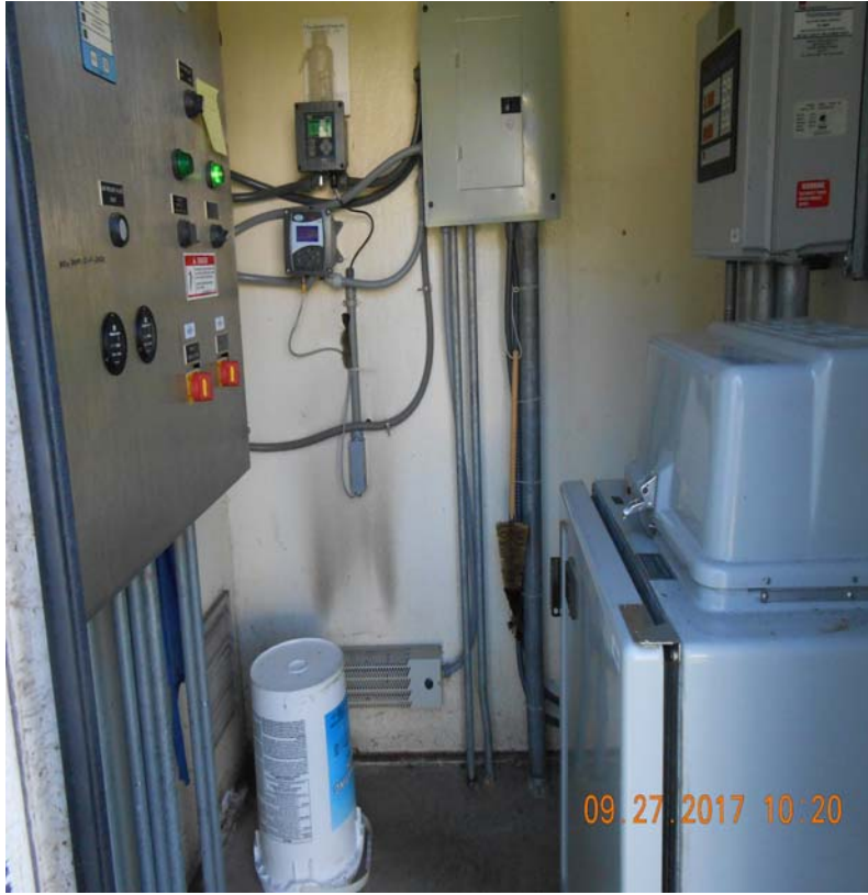
Control Panel in UV Control Building
