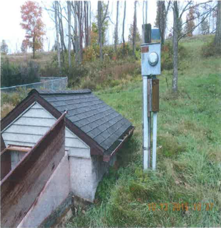
Well House (Exterior) Tank (Back Ground)
