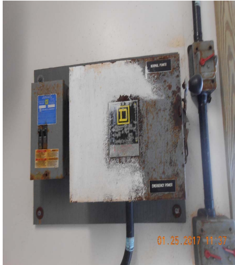
Well # 2 Control Panel
