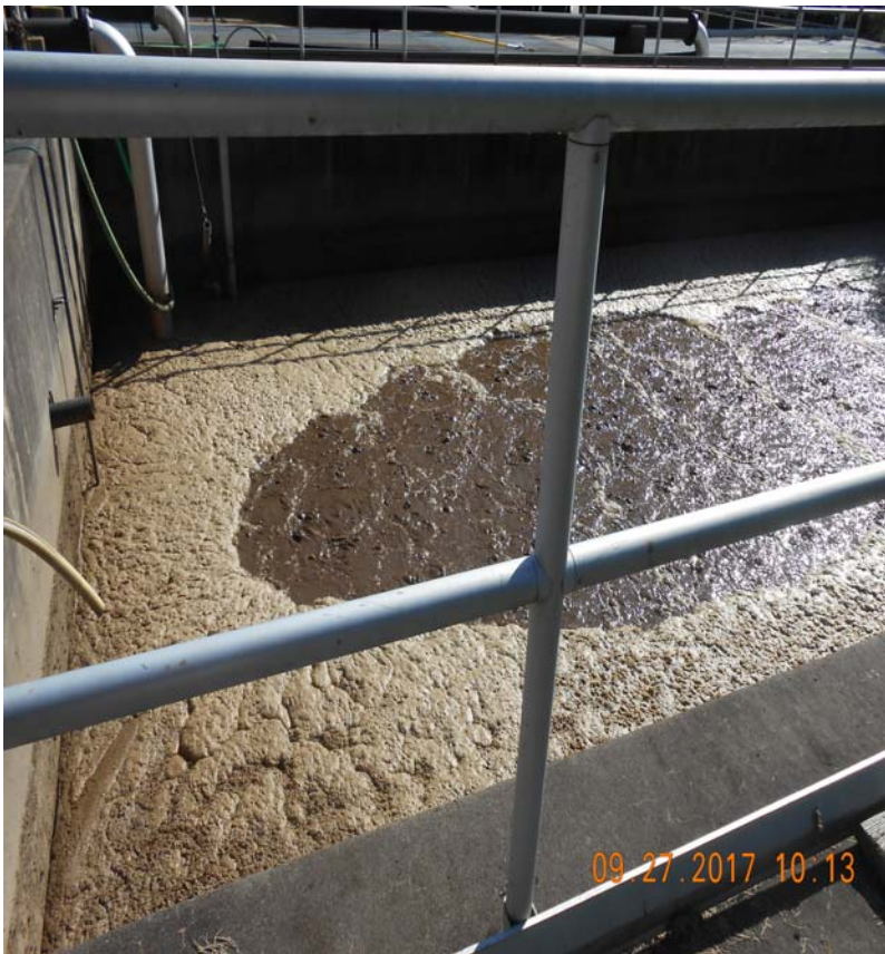
Sludge Holding Tank
