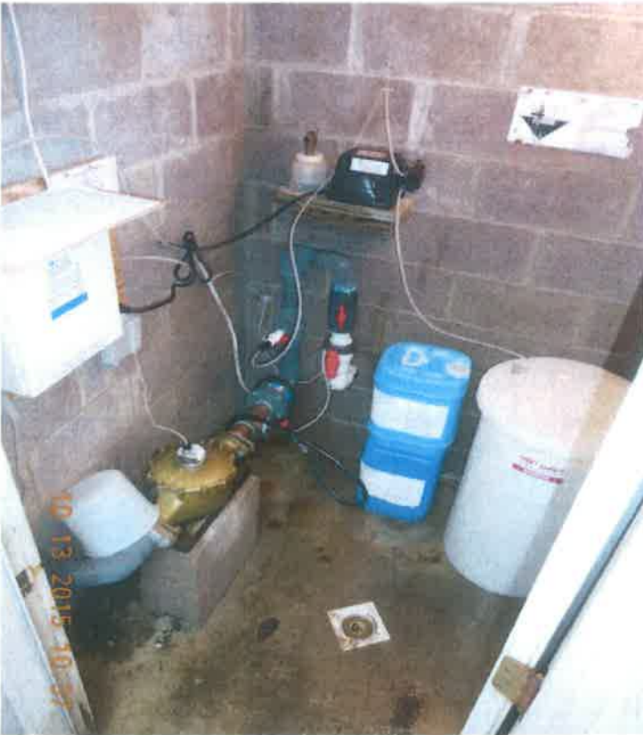
Well House (Interior) Chemical Feeder
