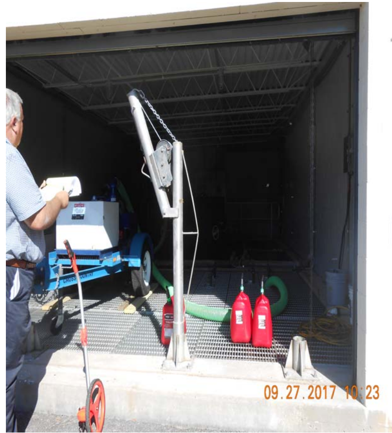
Back Wash Pumps
