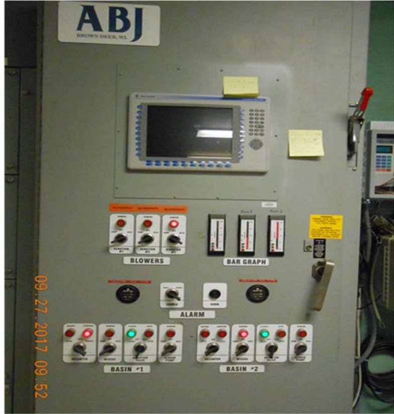
Blower Control Panel
