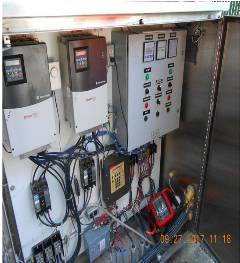
Control Panel for 940 Pump Station
