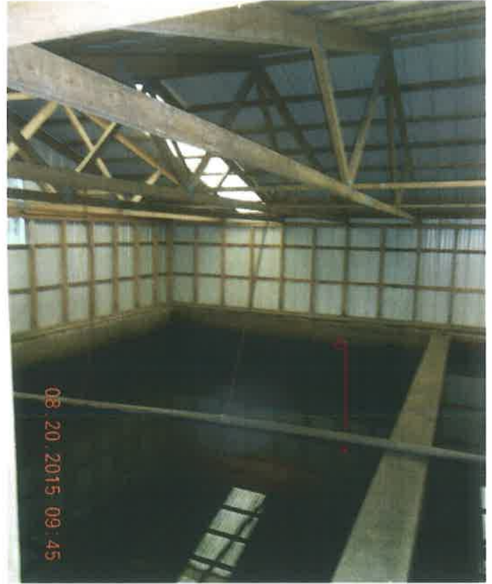
Inside Wash Water Building
