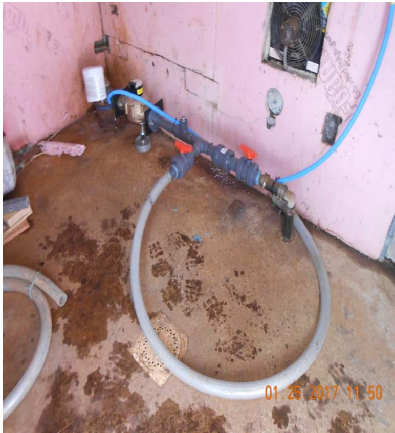
Interior Well House # 1
