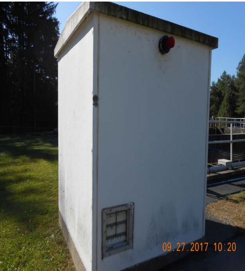
Control Building for UV Filters
