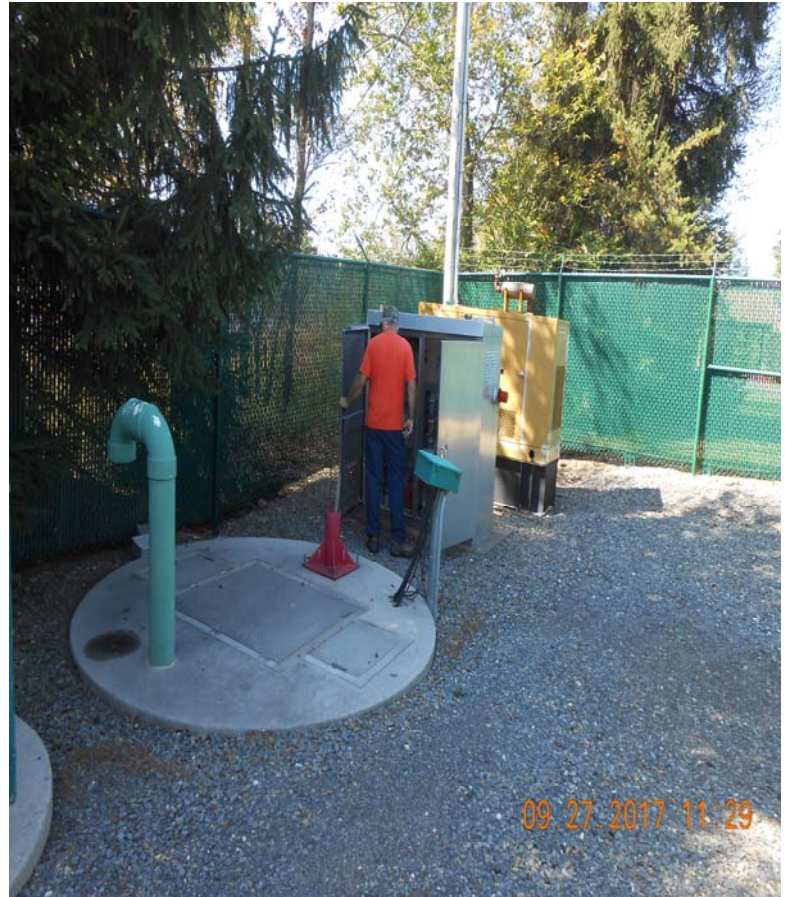
Fernridge Pump Station
