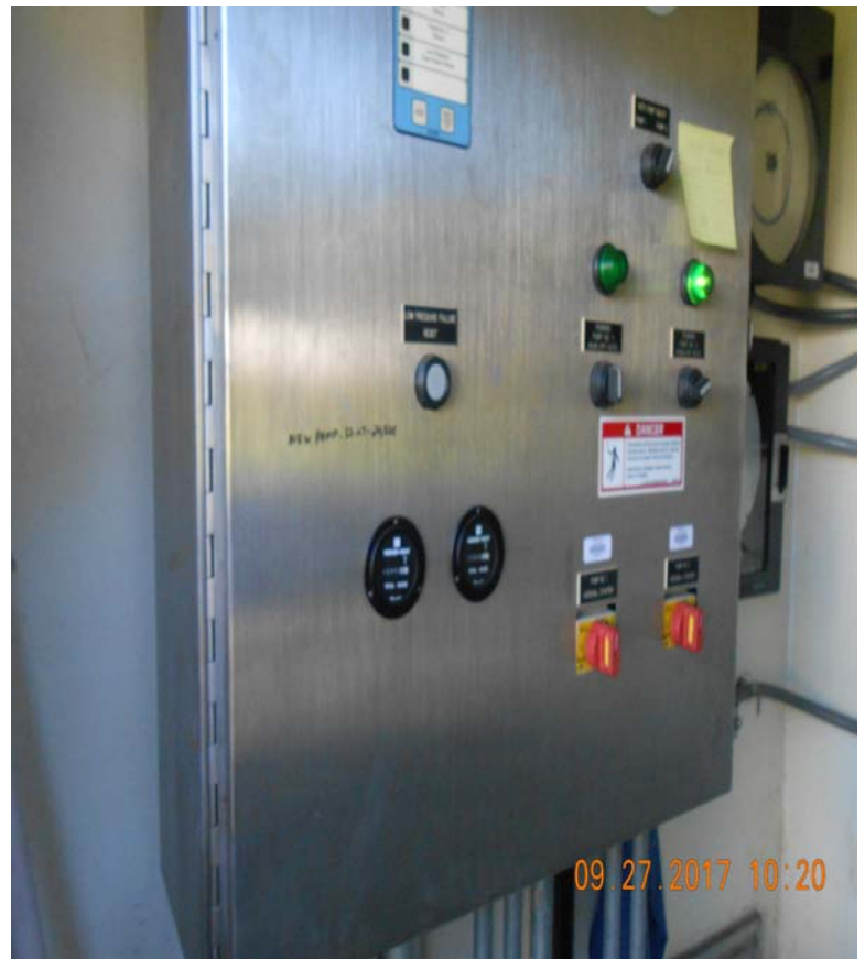
Control Panel in UV Control Building
