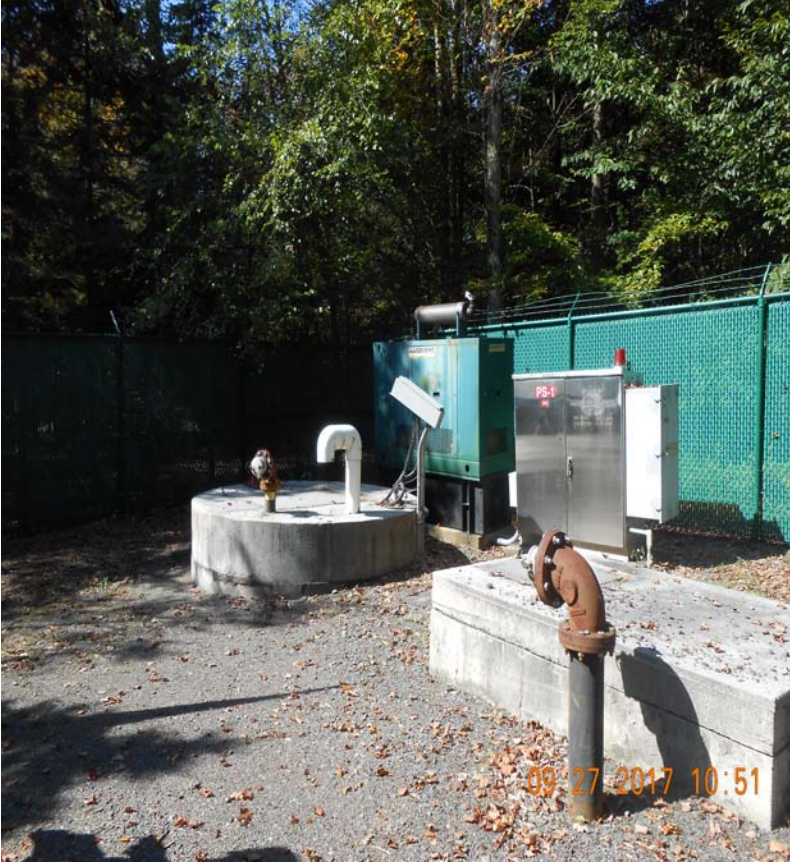
Lady Jennifer Pump Station
