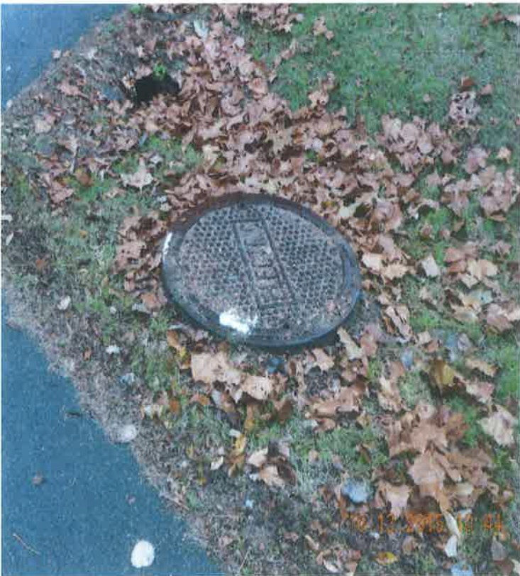
Water Manhole (Contains Pressure Reducing Valve)
