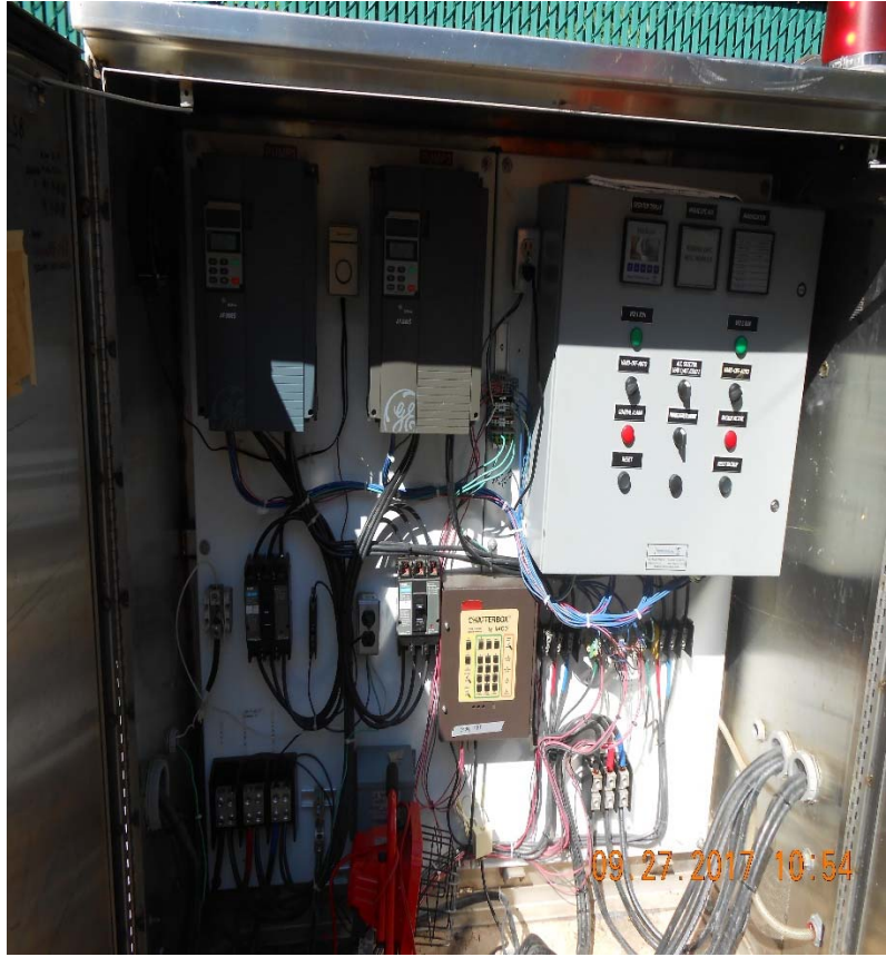
Control Panel for Pump Station #1
