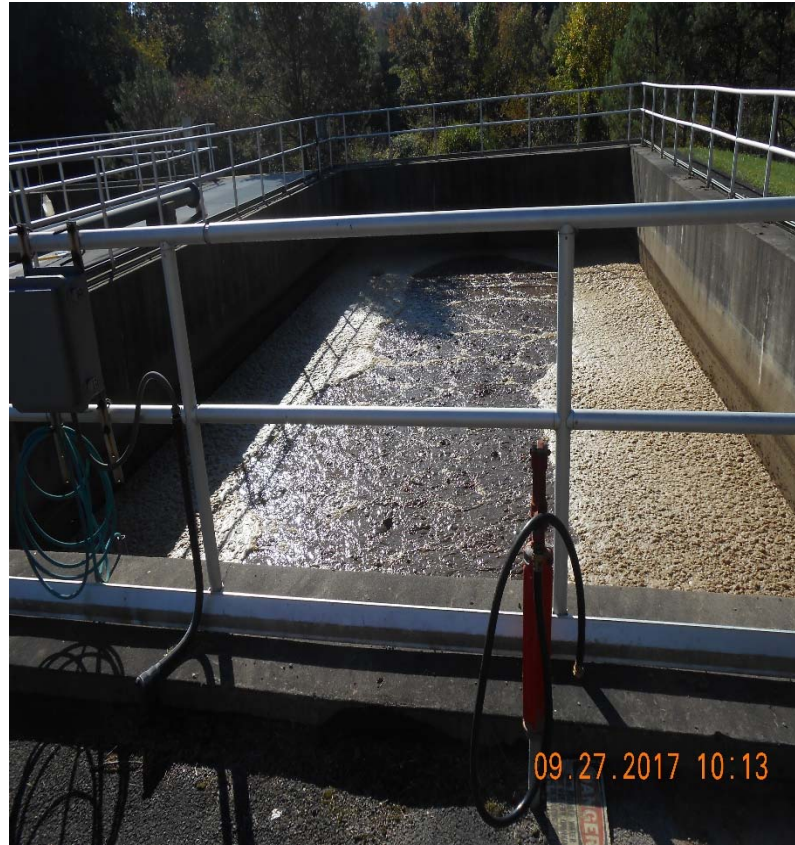
Sludge Holding Tank
