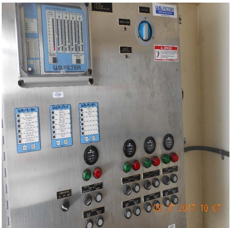
Control Panel for Submersible Pumps
