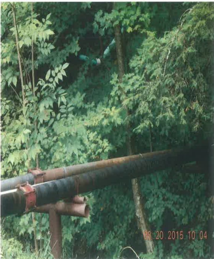
Water Lines from Wells
