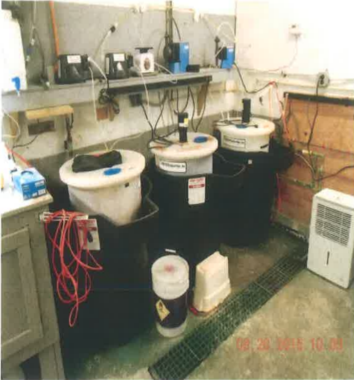
Chemical Tanks and Pumps
