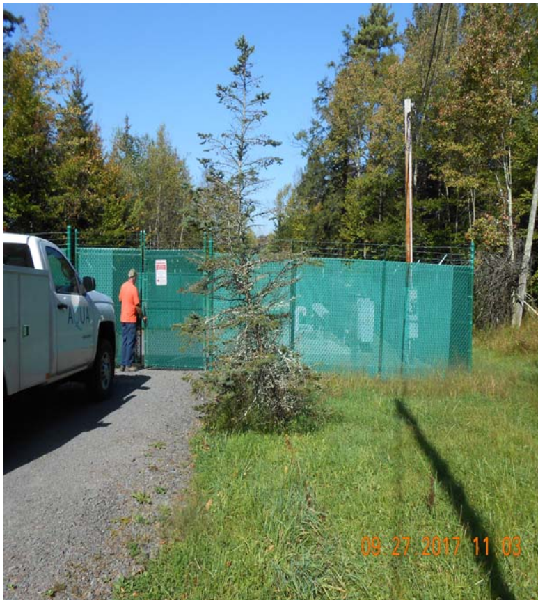
Pump Station #2 – Greenwood
