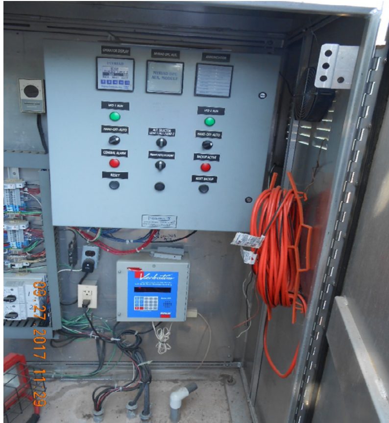
Fernridge Control Panel
