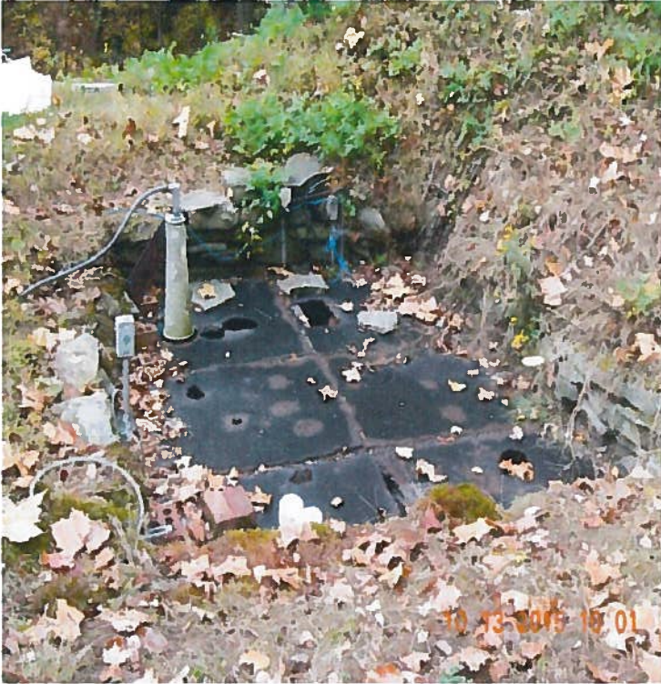
Chlorine Contact Tank
