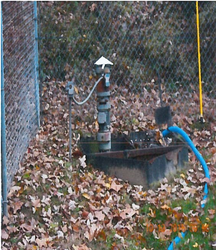
Grinder Pump (not in use)
