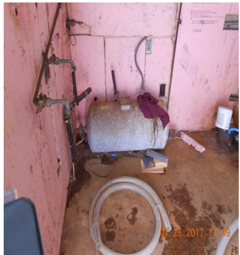
Interior Well House # 1
