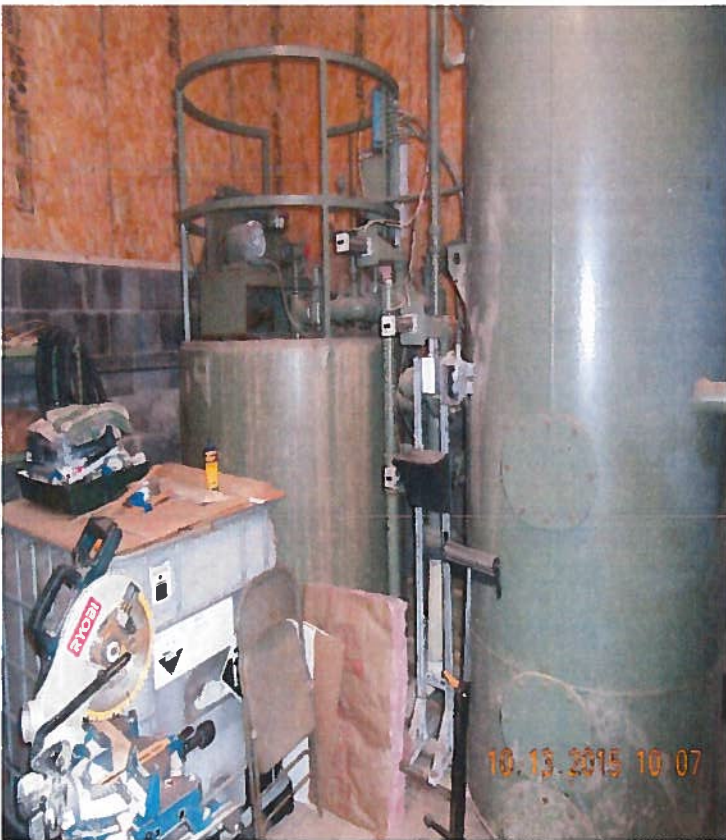
Sand Filters (Not used)
