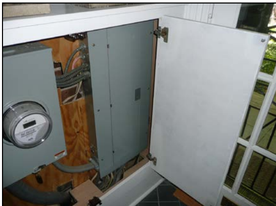
This interior electric meter is concealed in a narrow cabinet in the front hall.
