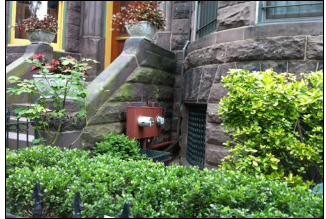
A utility meter installed below the top of a masonry stair and partially screened from the sidewalk by landscaping.
