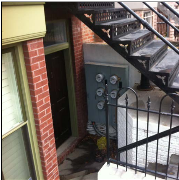
Electric meters within a basement areaway do not protrude into open space front yards and are consistent with the city’s public space regulations.
