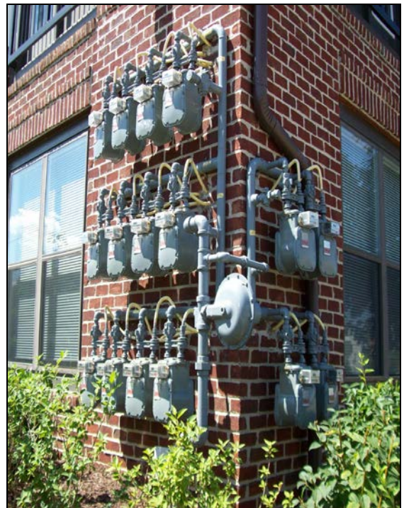
Installations resulting in three or more meters should be within an interior meter room or on a secondary elevation not prominently visible from the street.
