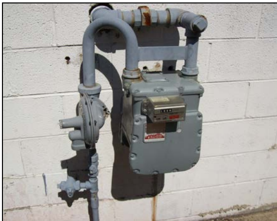
A single gas meter is typically not visually intrusive or difficult to accommodate on historic property.
