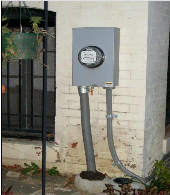
A single electric meter, as is still found on many Washington houses, is typically not obtrusive or difficult to accommodate on the exterior of the property.
