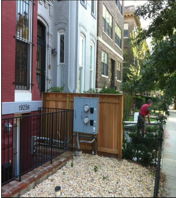
This meter box and solid fence protrude into the open space front yards in this block and are not consistent with the city’s public space regulations.
