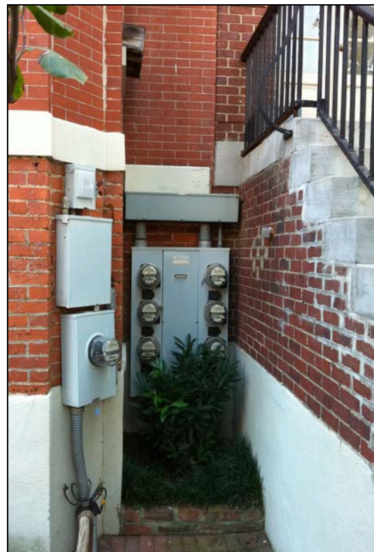
These meters were unobtrusively inserted between a projecting bay and the stairs to the adjacent property.
