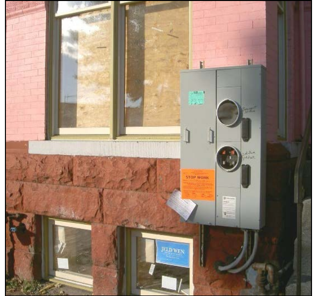
When increasing electric service or converting a property to multiple units, it is important to plan ahead for placement of the larger meter cabinet so that it doesn't detract from the property's appearance.
