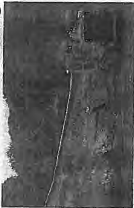
SENTINEL FILE Crews work on Sunoco's Mariner East 2 pipeline project in Silver Spring Township in 2017.
