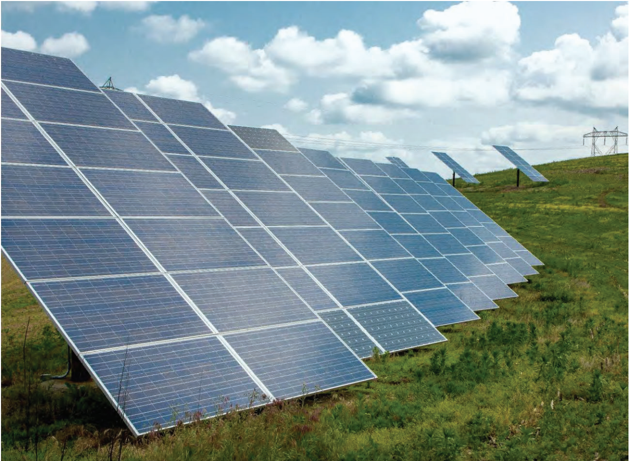
Solar panels in Germansville, Lehigh County
