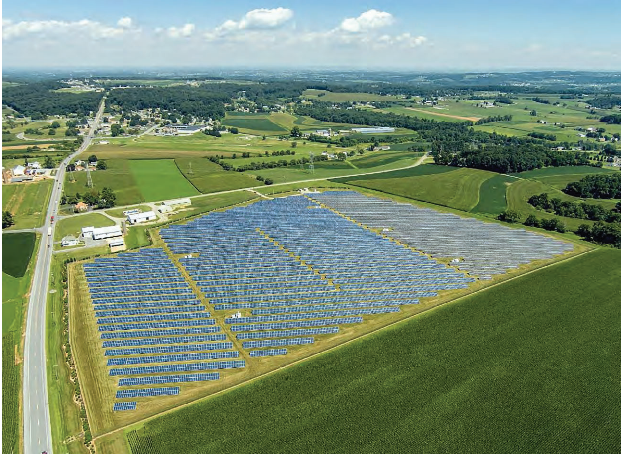
Community Energy's Keystone Solar Project, Radnor, Lancaster County
