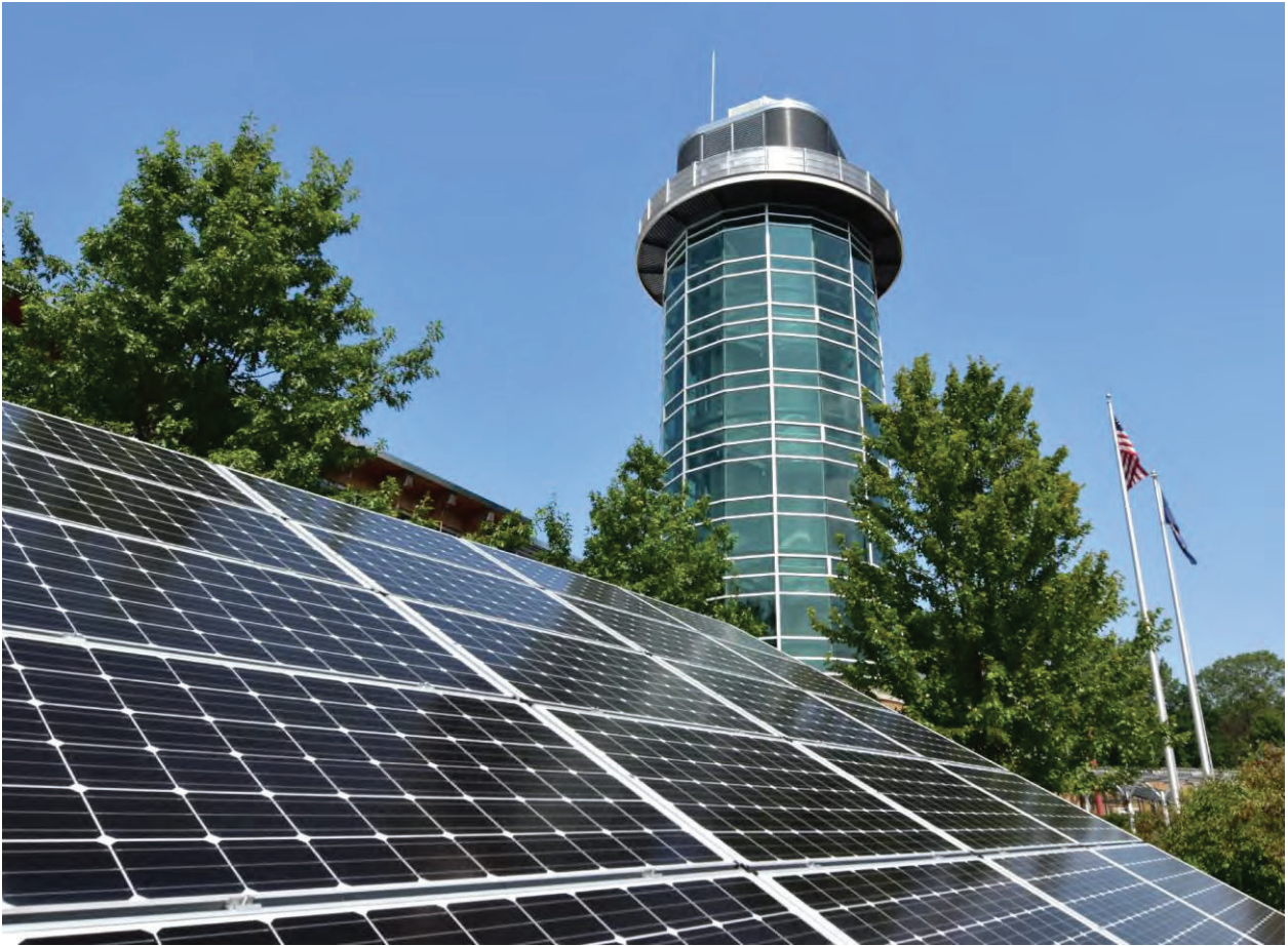
Solar panels at the Tom Ridge Environmental Center, Presque Isle, Erie County
