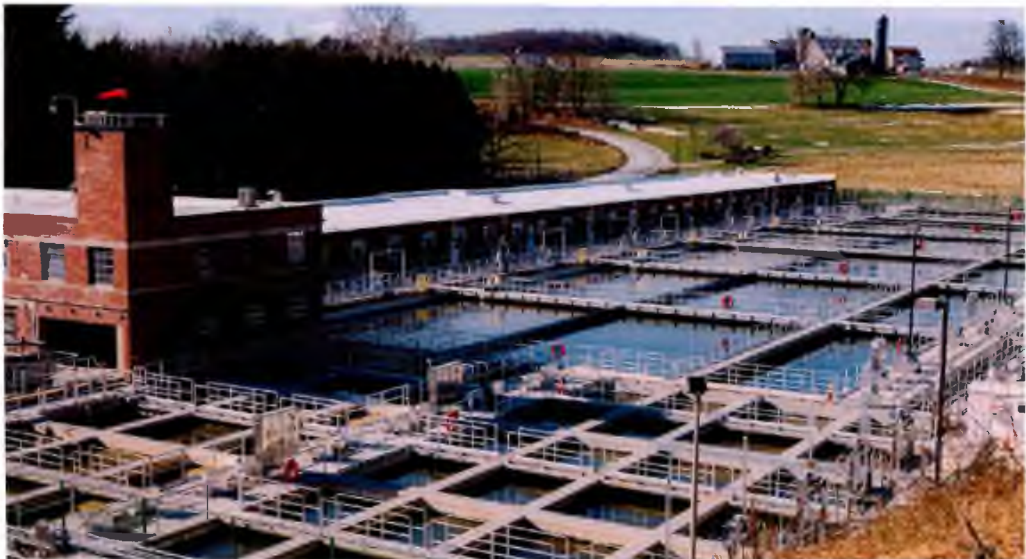
The outdoor conventional treatment pools at the Chester Water Authority (CWA) treatment plant in Nottingham, Pennsylvania.
