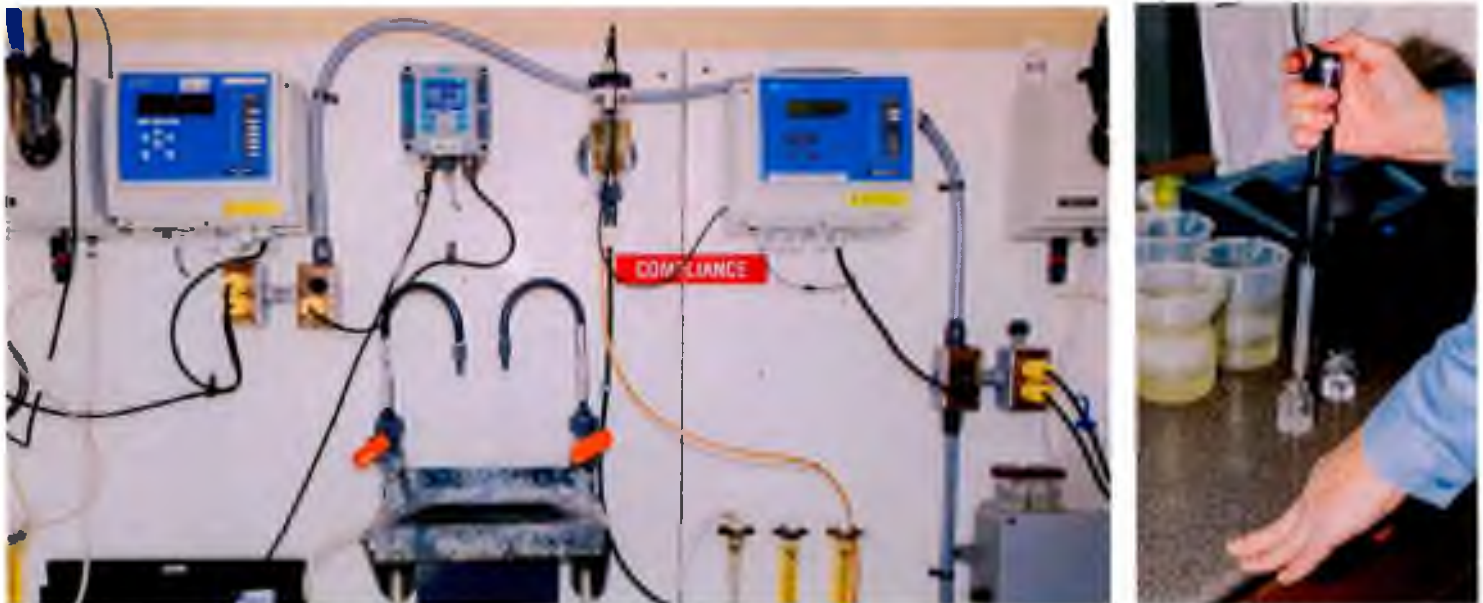
Left: Water analyzing equipment at the Chester Water Authority treatment plant. Right: Water being tested for chlorine residuals.
